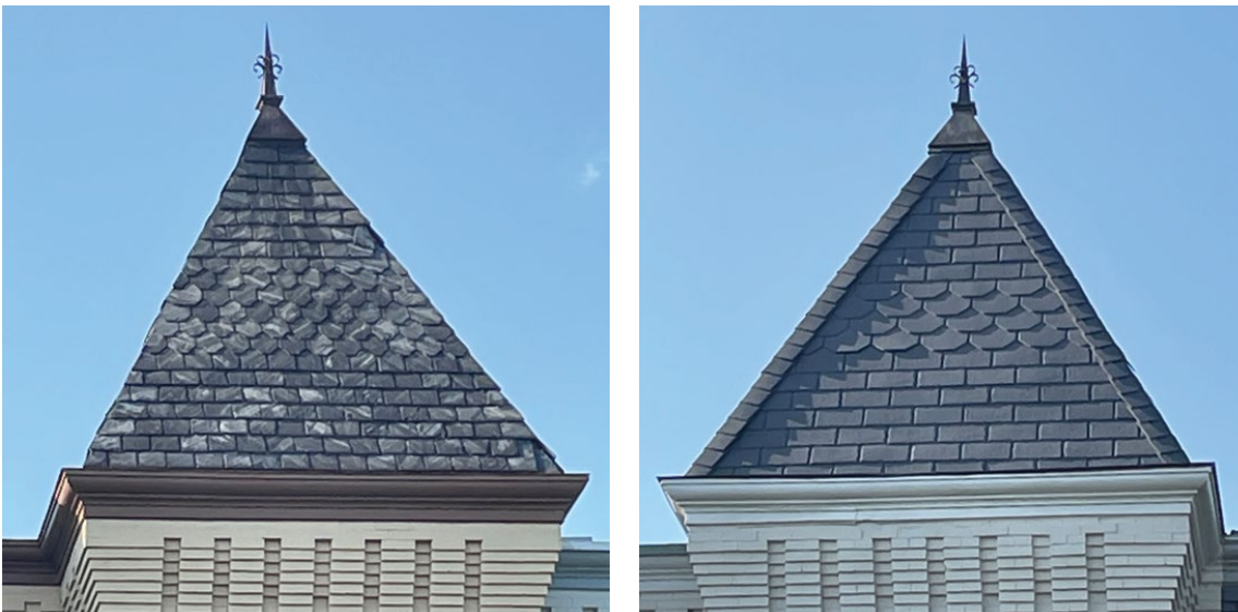
Figure 10. Polymer slates offer a choice of shapes but not sizes, limiting their ability to achieve a good visual match for some historic slate. With the size of the polymer slates (right) being nearly twice that of the historic slates (left), the scale of the entire feature is incompatibly altered. The molded edges of this material, which contribute to its ability to replicate slate, would be lost if each shingle was resized by cutting. Photo: John Sandor, NPS.
