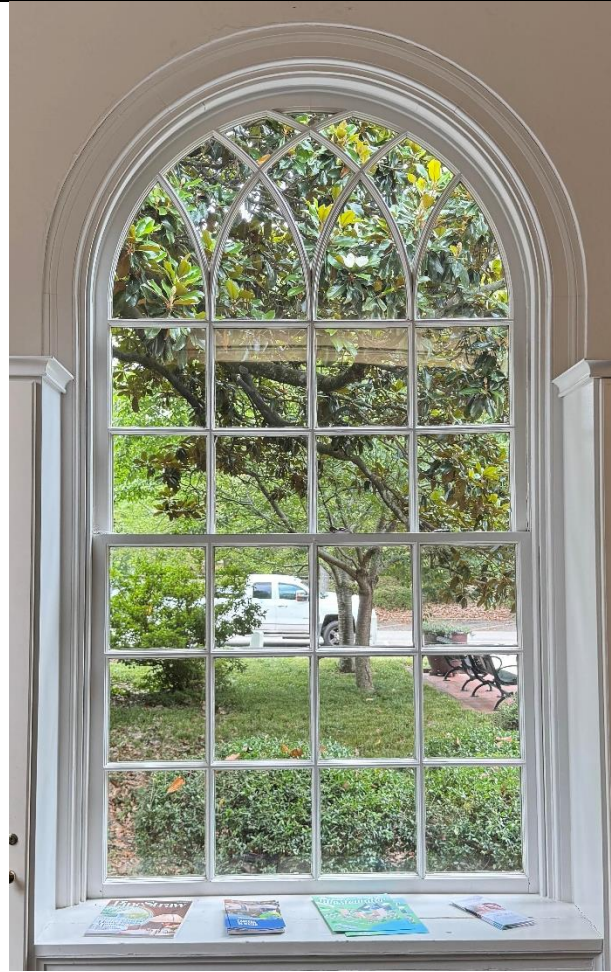
Figure 3: Existing Window View of one window from interior, Provided by the Town of Southern Pines (20 June 2025).
