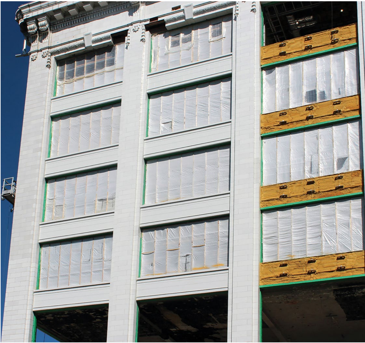
Figure 18. Missing historic terra cotta spandrel panels on all floor levels were recreated utilizing glass fiber reinforced concrete (GFRC) replacements. New spandrels were fabricated as individual components and attached with metal terra clips between historic terra cotta piers. Photo: Kris Frail, Dewberry.
