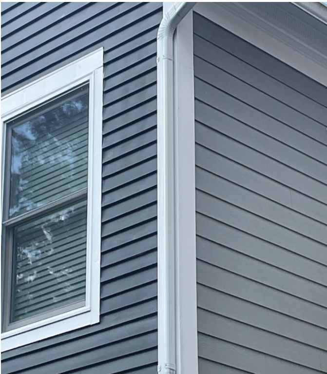
Figure 11. The thickness of the wood siding on the front (left) creates a deeper shadow line than is achieved with the fiber cement siding used on the side (right) elevation. While the exposure can be adjusted, fiber cement siding is not available in a matching thickness. Photo: John Sandor, NPS.
