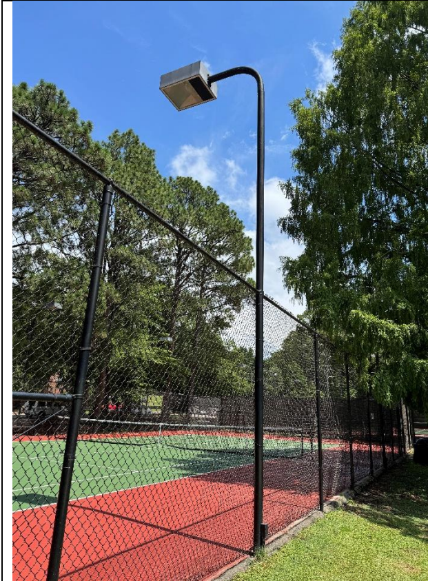
Figure 7: One of several existing light poles adjacent to the tennis courts to be replaced. (Photo provided by staff)
