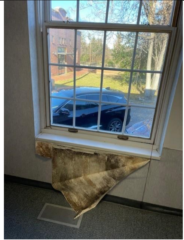
Figure 7: Interior Window Damage (Two)
