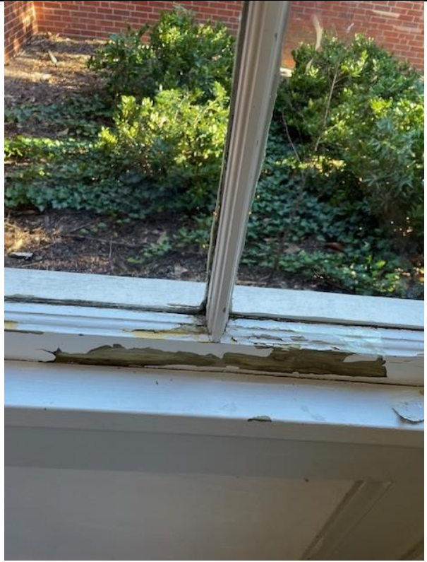
Figure 9: Interior Window Damage (Four)
