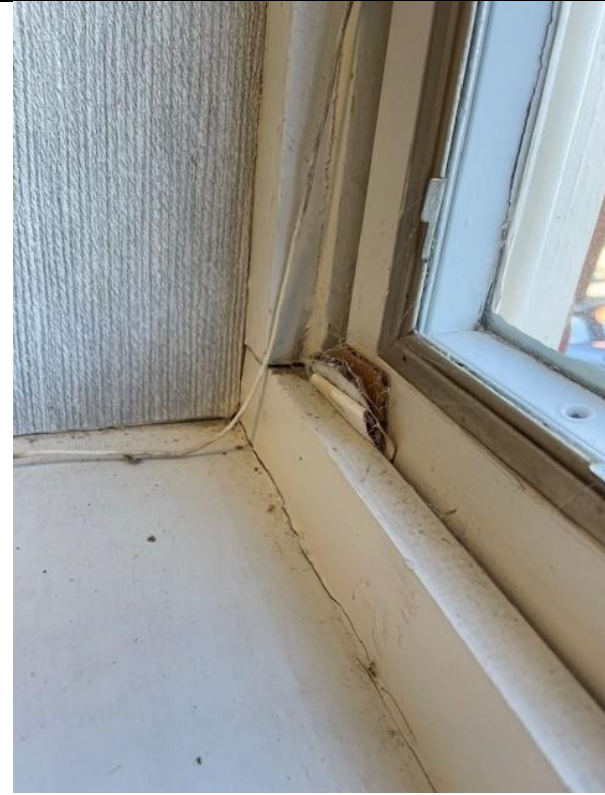
Figure 6: Interior Window Damage (One)
