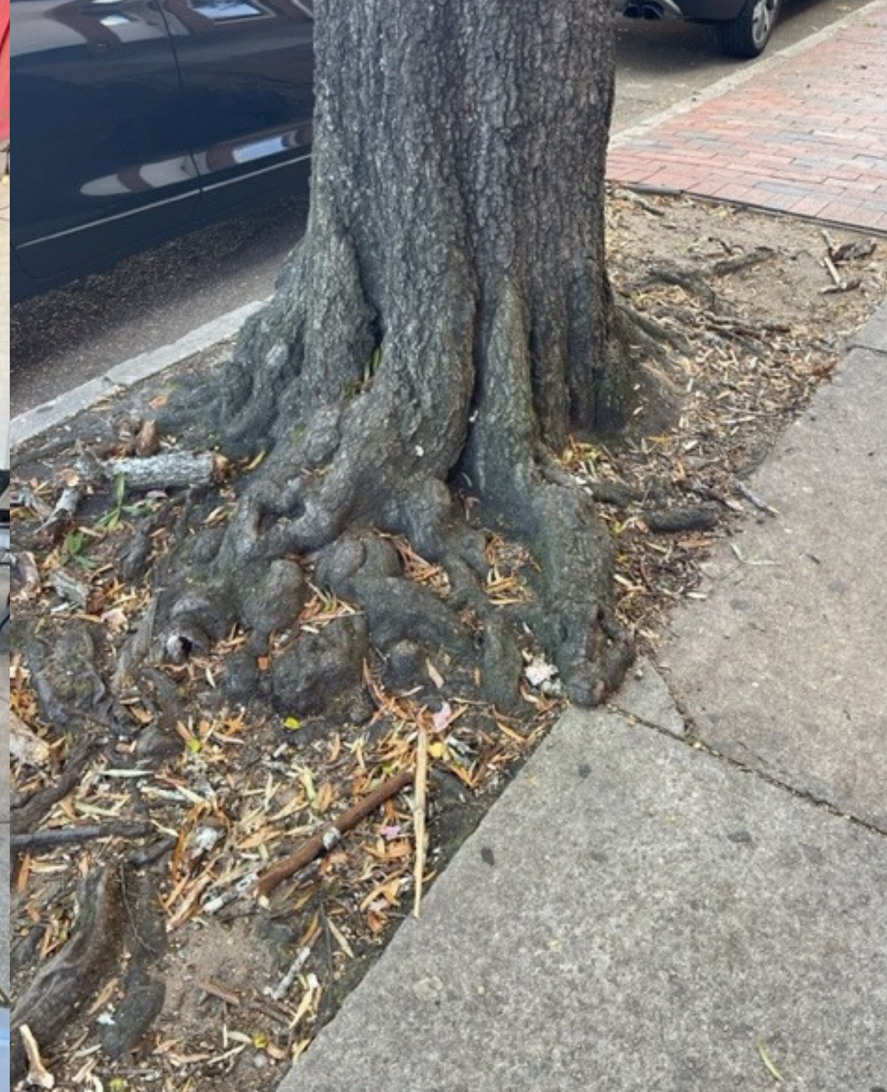
Roots lifting up the sidewalk
