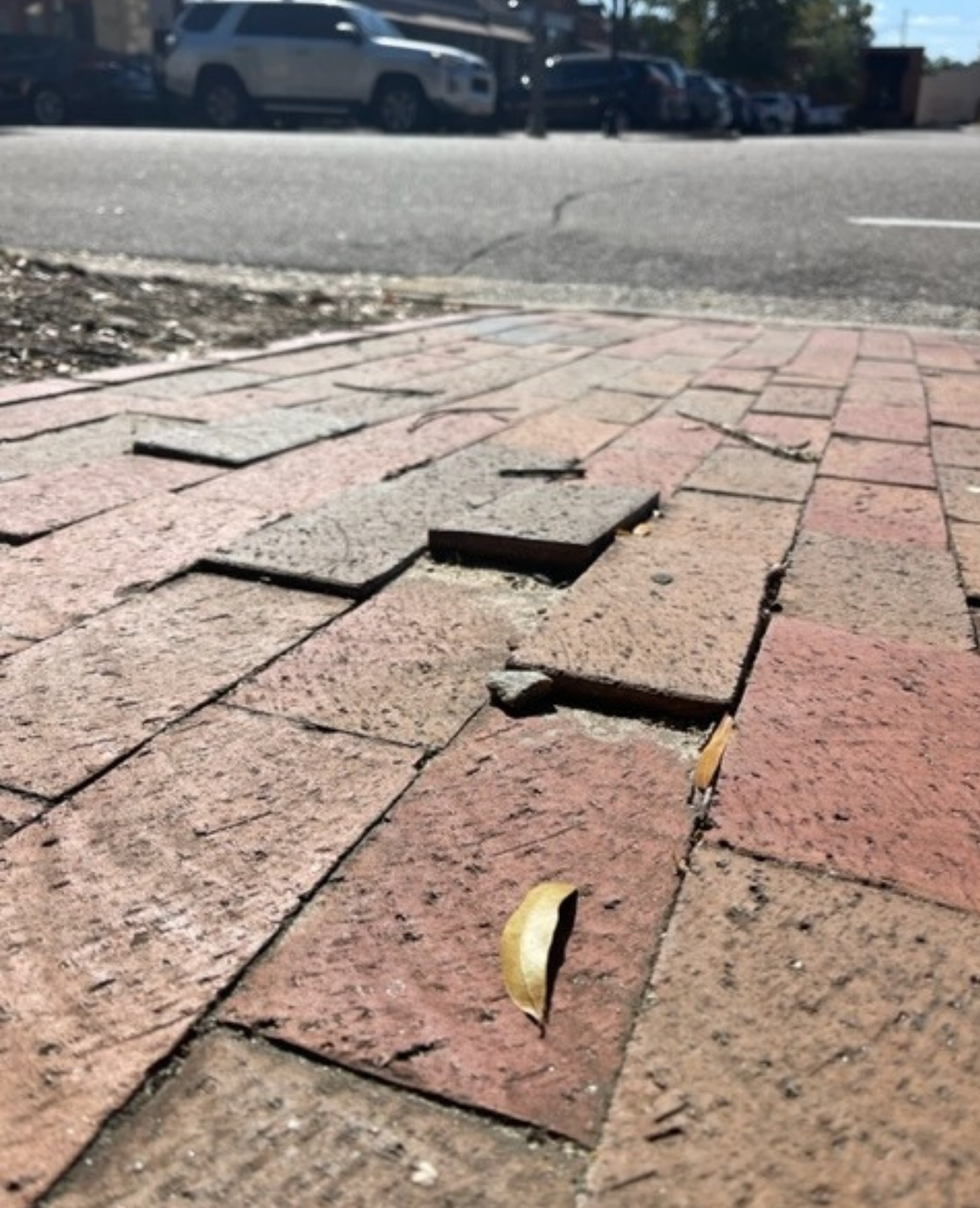
Overgrown roots lifting up brick
