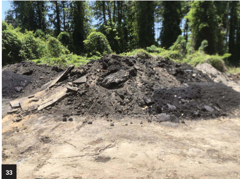
Asphalt rubble piles in materials storage area located in the east-central portion of Area 2
