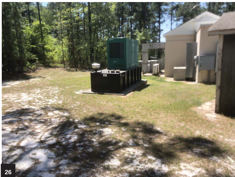
Emergency generator and diesel tank in Time Warner lease area
