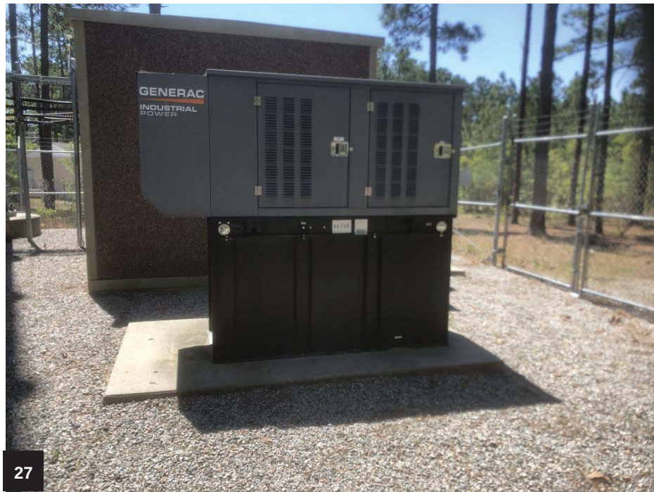
Emergency generator and diesel tank in NC Highway Patrol lease area in northwest corner of Area 2
