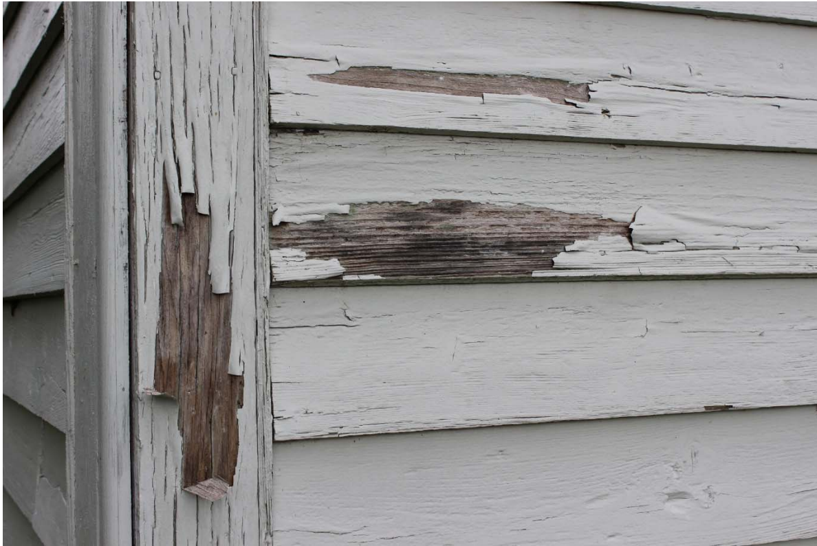
Fig. 3. Decay and paint failure on 6-year old replacement siding and trim on a historic Rosenwald School.
