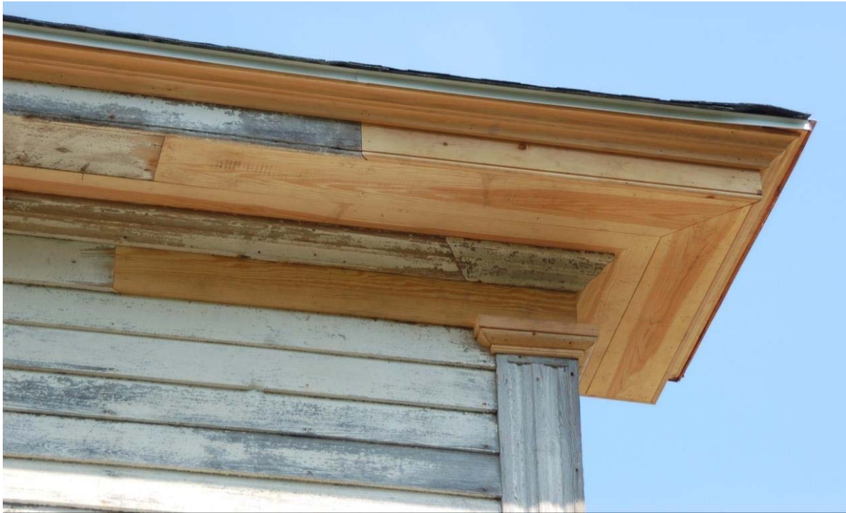
Fig. 4. Cornice repairs on a mid-19 th -century Pitt County farmhouse. This corner was decayed due to long-term roof leaks.
