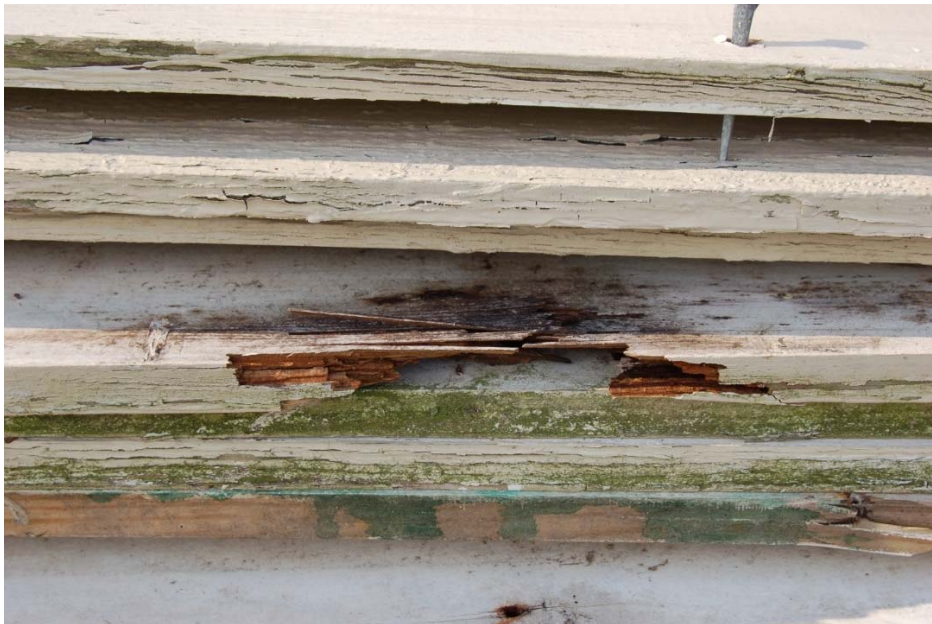
Fig. 2. 10-year old decayed replacement siding.
