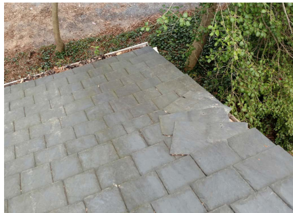
4.6 Damaged slate tiles
