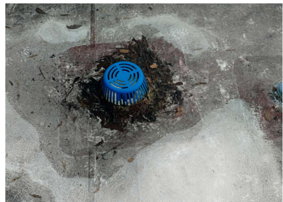
4.3 Clogged internal drain
