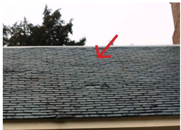
4.3 Missing slate tile
