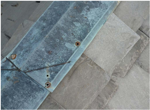
4.7 Missing fasteners and holes in the copper ridge flashing
