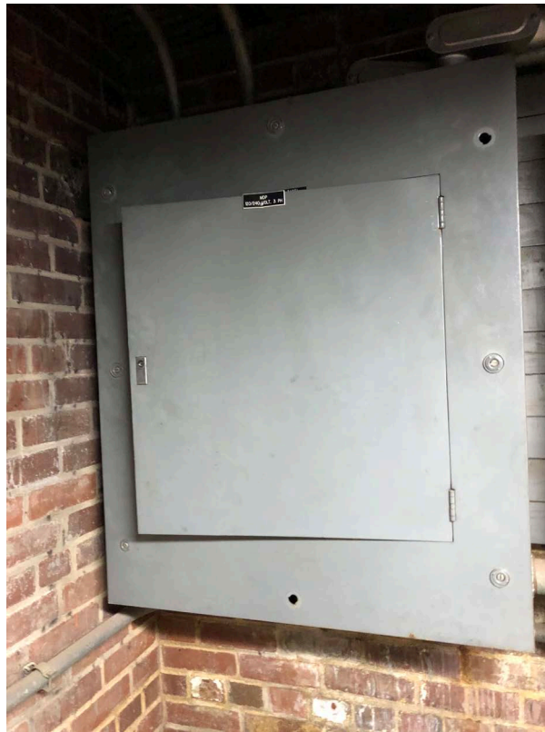
Main Distribution Panel
