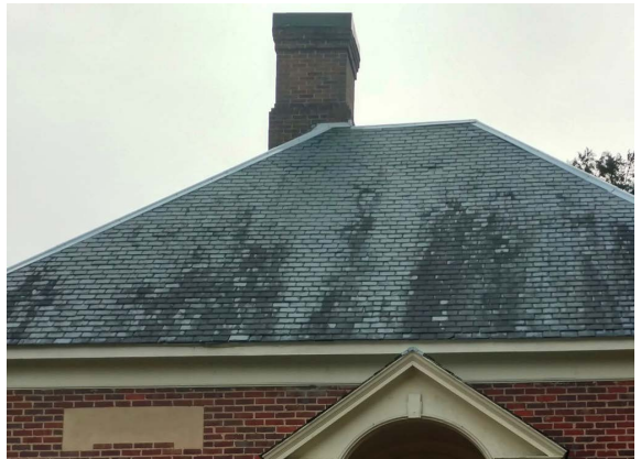
4.2 Missing and damaged tiles
