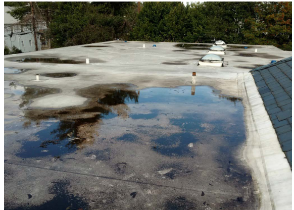
4.2 Ponding and staining on single-ply roof
