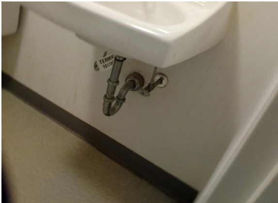
7.2 Piping under the sink
