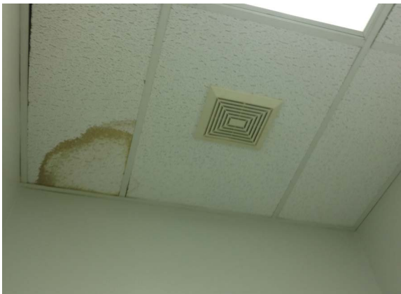
5.6 Stained ceiling tiles
