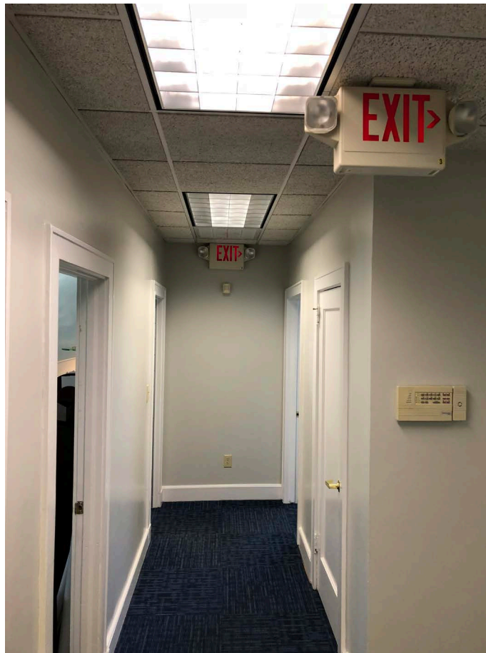
Typical Exit Sign and Battery Pack
