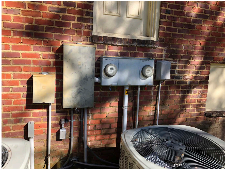
Service and Panels
