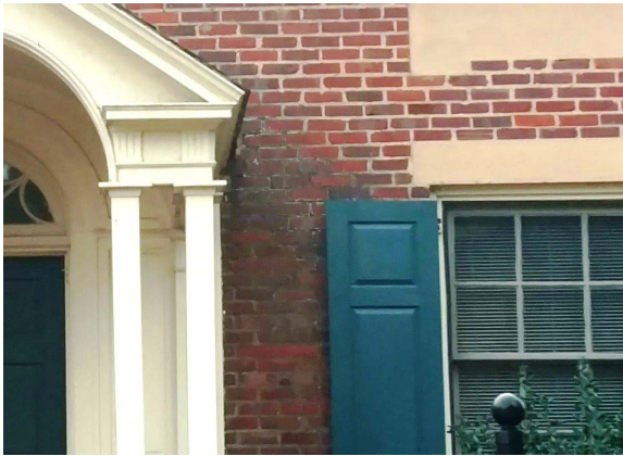
1.5 Typical staining on the brick
