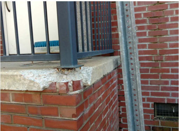
1.5 Damage concrete landing and rail attachment
