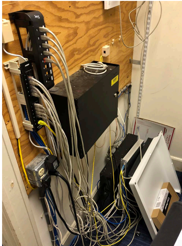
Main Data Room
