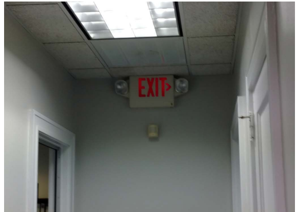
6.2 Exit signs and lighting
