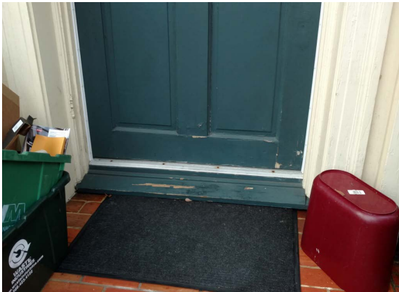
2.3 Deteriorated painting on the front door
